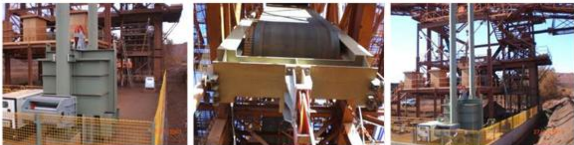
Image of Maintenance Shut-Down Related Project Planned and Executed Successfully During a series of Shut-Downs at Greater Paraborde Mines, WA, Australia, 2007.
